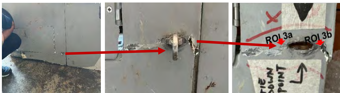
Figure 38. RH Wing – Tie-Down Ring and Man-Made Hole
