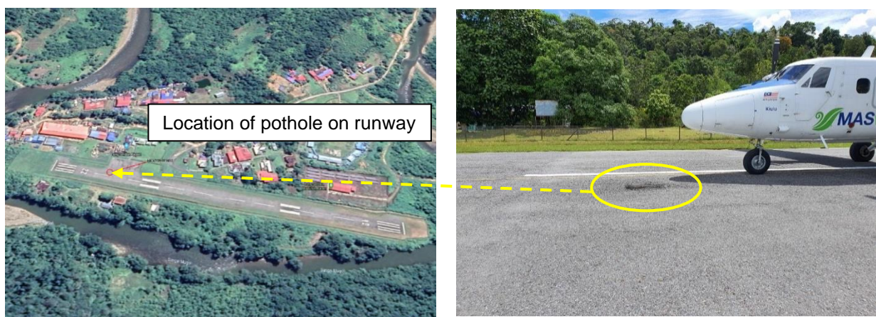
Figure 17: Aerial view of the location of the pothole and location of the pothole on the runway close to centreline
