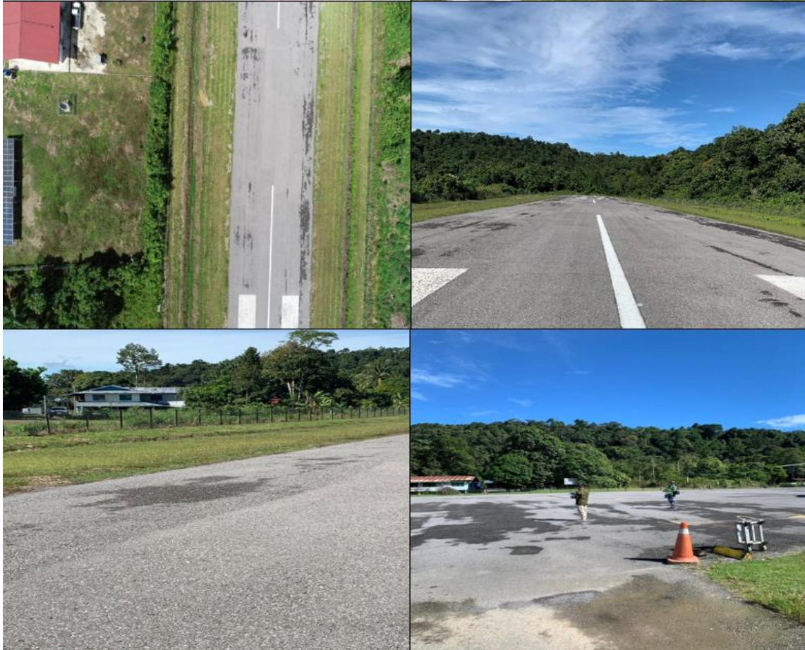
Figure 32: Water bleeding (black spots) distress occurrence on Long Seridan runway
