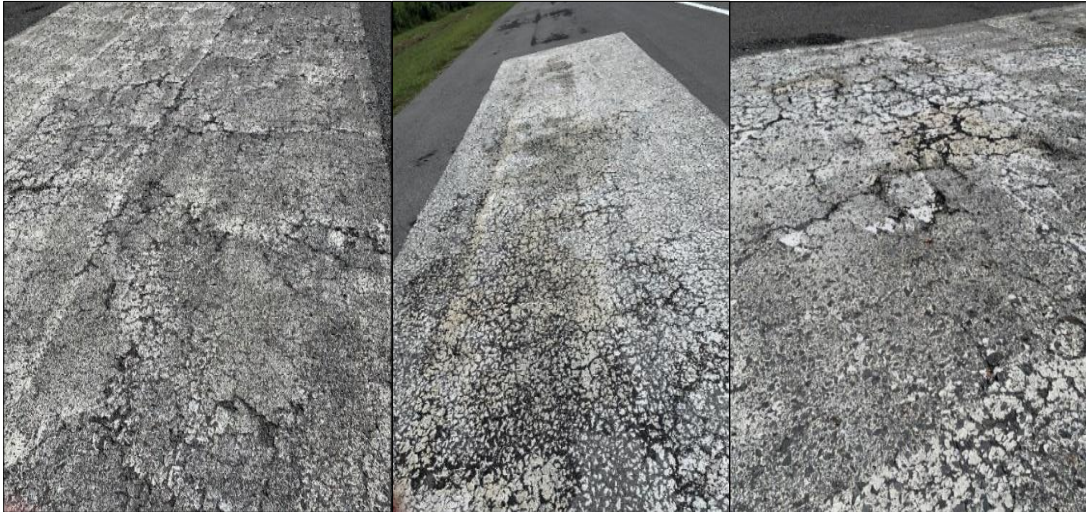
Figure 33: Cracking distress on Long Seridan runway
