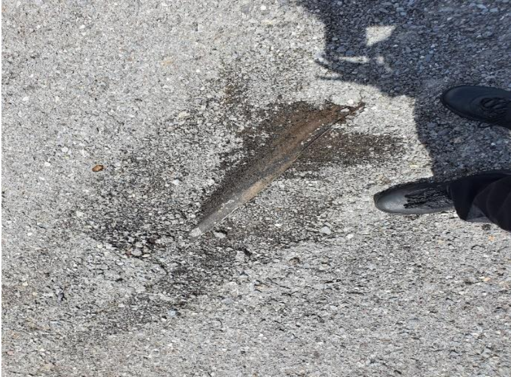
Figure 18: Close up view of the pothole. The pothole appears over time due to disintegration in asphalt pavement.
