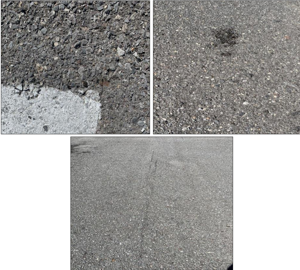
Figure 35: Polished aggregate distress on Long Seridan runway
