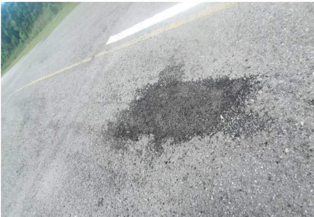
Figure 19: Repair carried out by Long Seridan staff using 'Cool Mix Asphalt'. Asphalt aggregate is observed to be loose and uneven.
