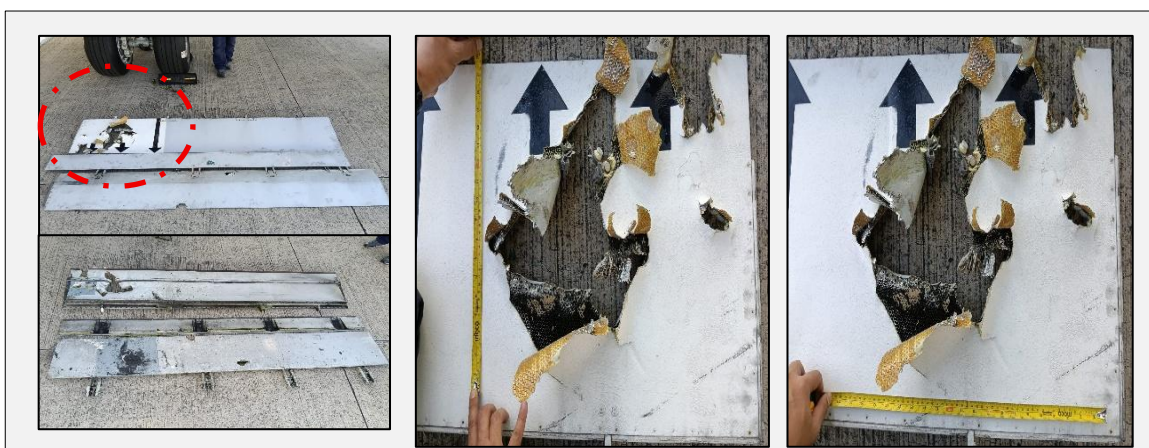
Figure 8: RH Ground Spoiler No 5 Ruptured
