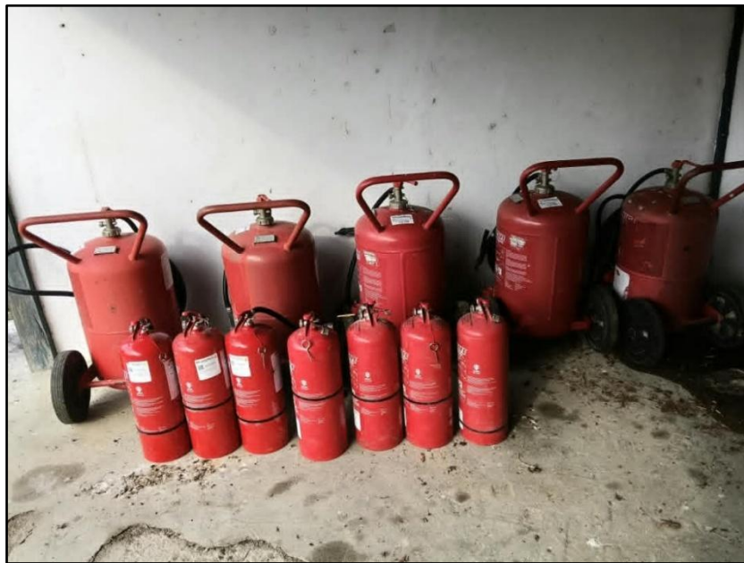
Figure 8: Dry powder fire extinguishers available at Long Lellang STOLport and used during the emergency response
