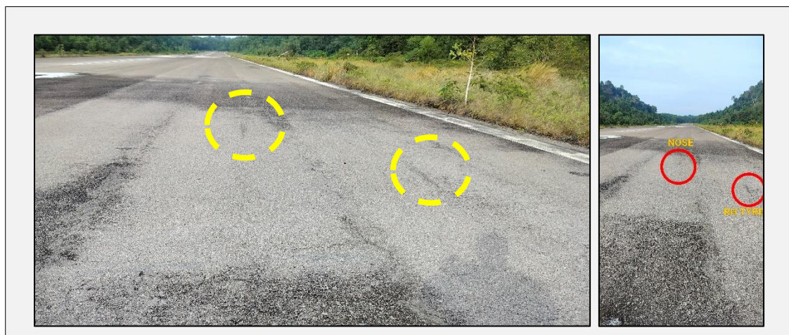
Figure 1: Nose and RH Main Landing Gear tyre marks were observed on Runway 22
