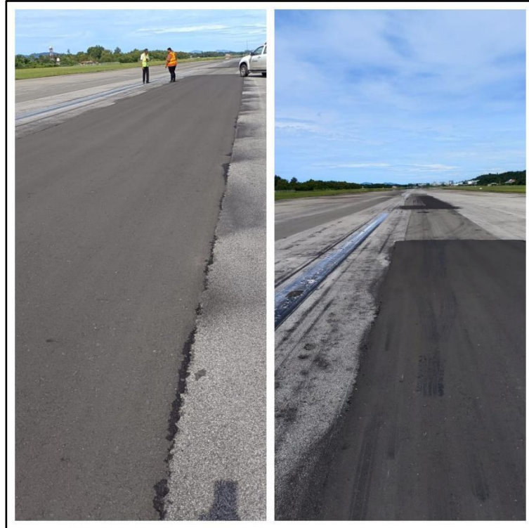
Figure 7: New big patch was applied but the joint at the side between the new and old started to dislodge gradually
