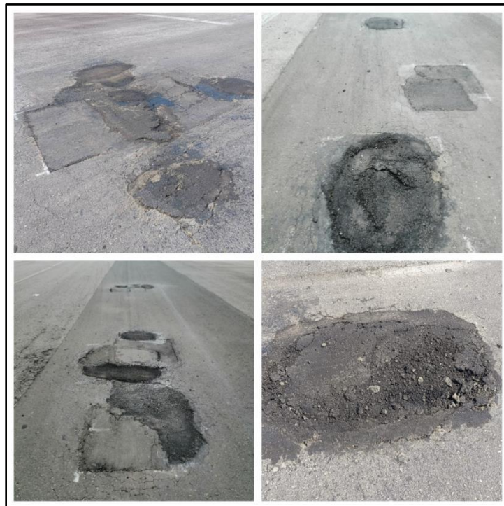
Figure 6: Peeled-off runway surface from temporary patchwork
