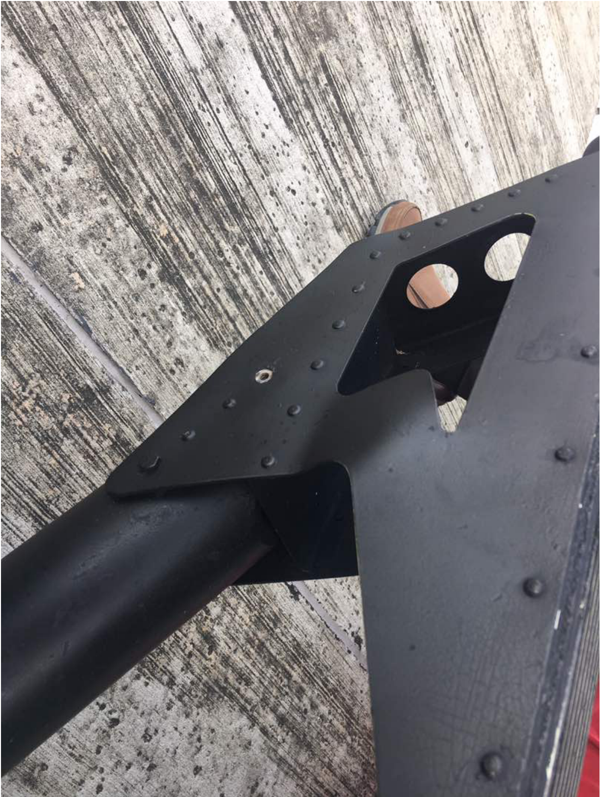
PHOTO 07 – Skid Pulled Rivet
