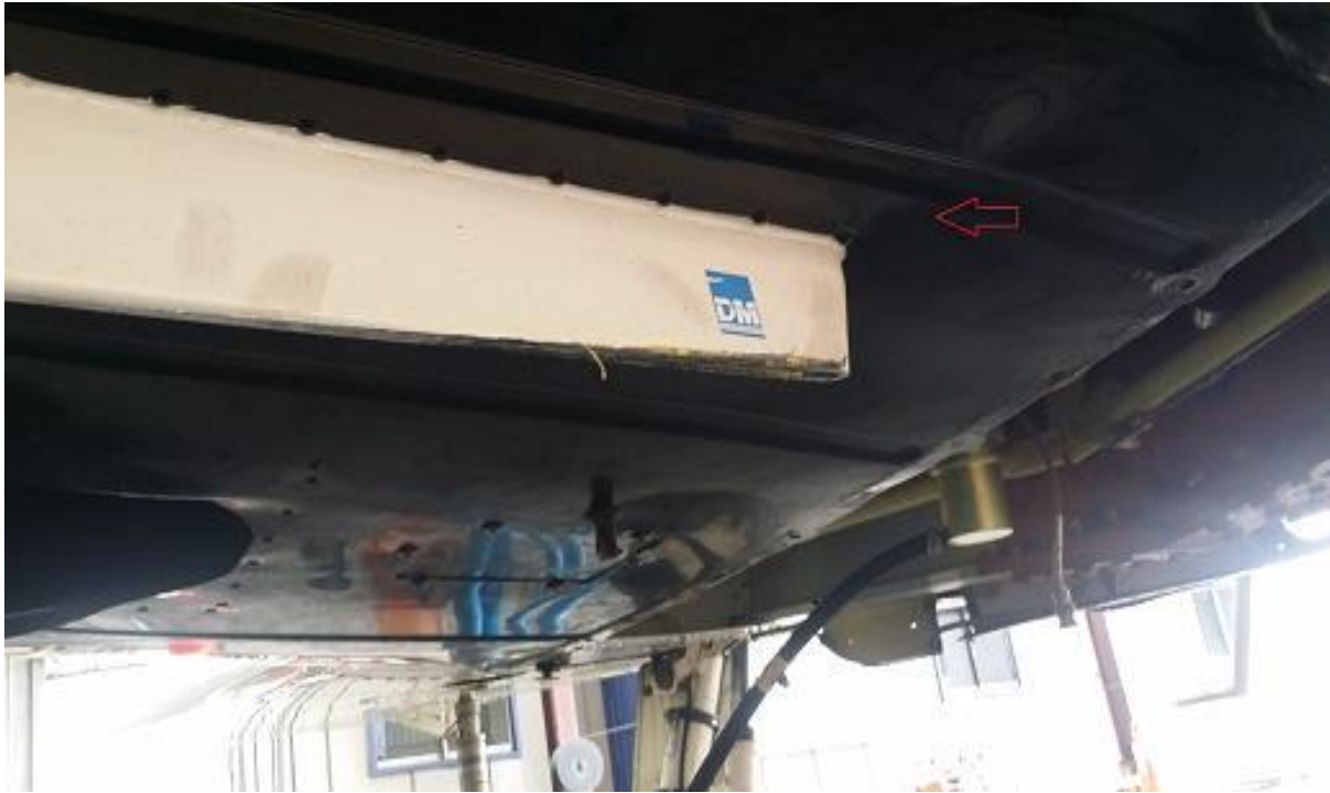
Figure 11 – Antenna attachment area dented
